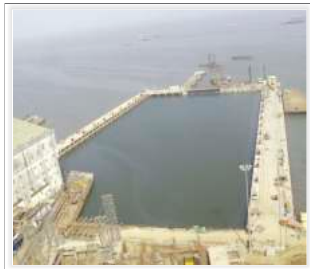
KBL's Impounding Pumphouse at Mazagon Dockyard Wet Basin
