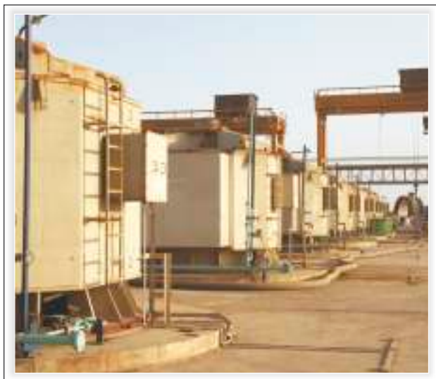
Concrete volute pump ready to start at Coastal Gujarat Power Limited, Mundra
