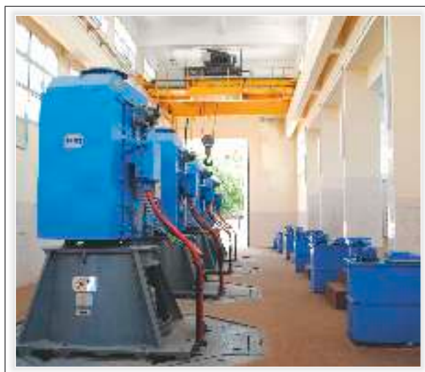
Pumping station at Benban, Egypt
