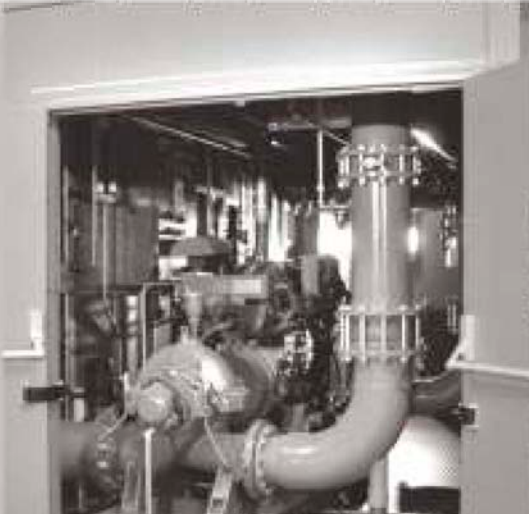
Kirloskar Containerised Fire Fighting Set
