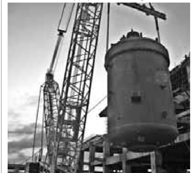
Erection of 90 MT Reactor for Polypropylene Unit of Phase III of OIL Refinery project for MRPL Mangalore, Karnataka
