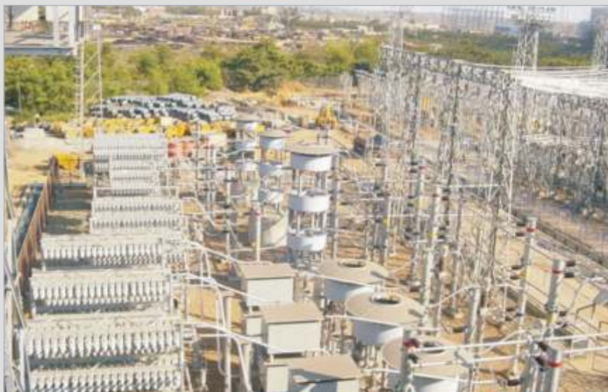
SVC: Improving performance levels by controlling voltage flicker and current distortions
