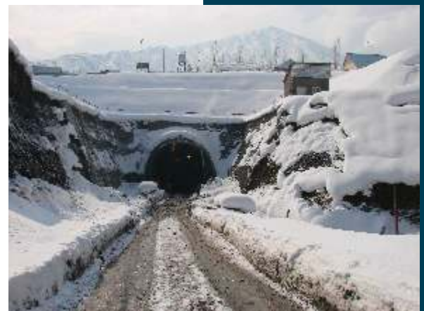
Design and construction supervision for 10.6 km long railway tunnel across Pir Panjal range, J&K State
