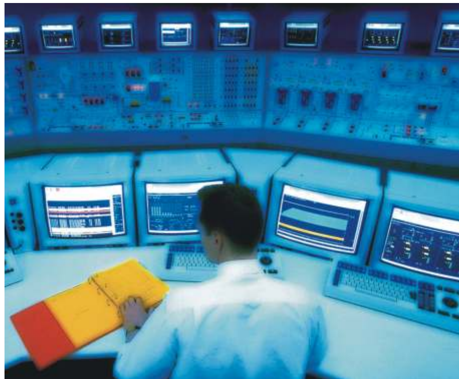
AREVA T&D supports the SmartGrid revolution through the use of IT technology with smart integrated solutions from Equipment to Central Markets
