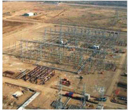
AREVA T&D India is implementing Electrical Balance of Plant (E-BOP) and equipment for Essar Power Plant projects in Gujarat and Madhya Pradesh
