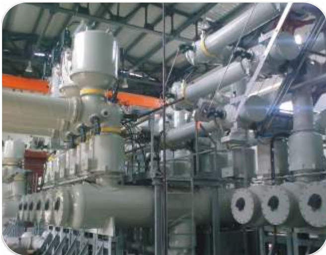
Successful commissioning of 400 kV indoor GIS substation for Lanco Kondapalli, an Independent Power Project (IPP) located near Vijaywada in South India
