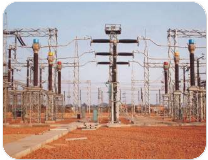
First OSKF 420 kV CT: Commissioned for Jindal Steel & Power at Angul, the largest integrated steel project in Orissa
