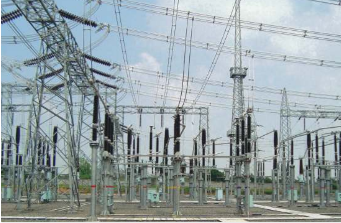
The 400/230 kV AIS substation at Pugalur. Termed the most modern substation, this project is first of its kind for AREVA T&D with products sourced from its various manufacturing facilities
