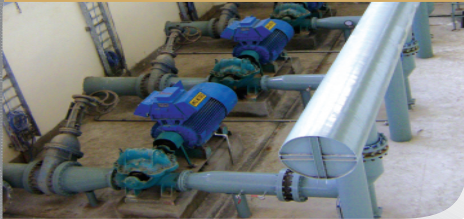
Ash Water Recirculation Pump House
