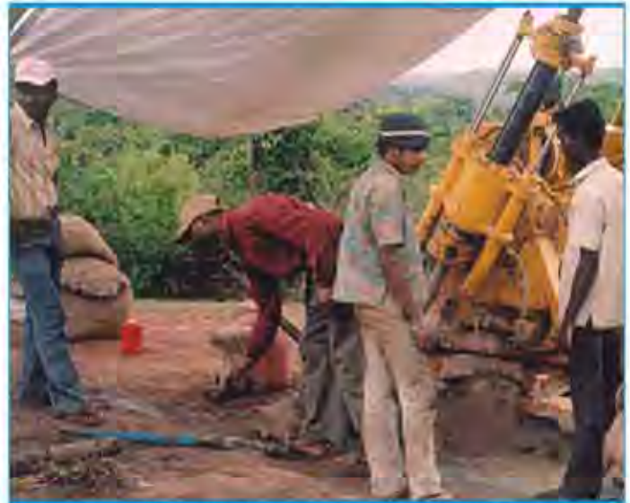
Geo-technical investigations for underground storage of LPG and crude oil in rock cavern projects, Vizag and Mangalore
