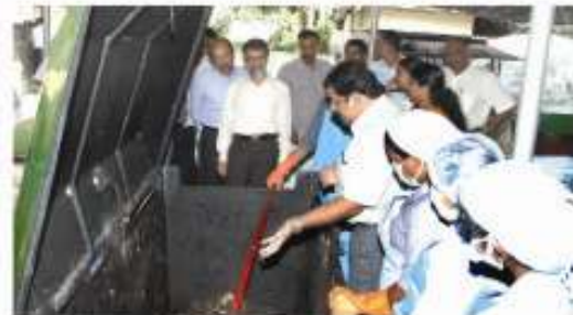
CSL Solid Waste Management system at Govt. Hospital, Ernakulam
