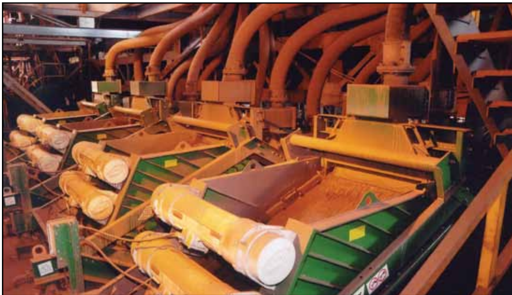
New Secondary (Derrick) Screen in operation
