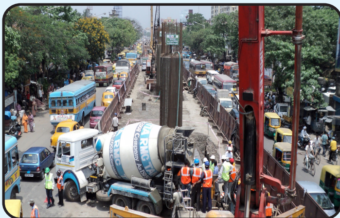
Aerial view of construction of Metro Viaduct in Jokha - Mominpur Section of Kolkata Metro
