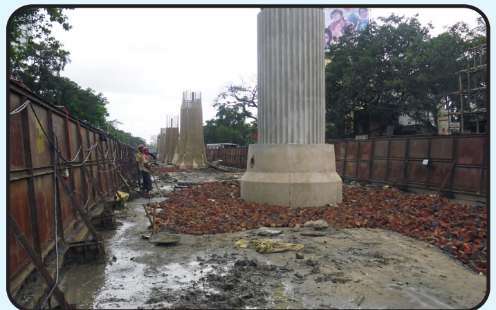
Isometric view of under construction piers in Jokha - Mominpur Section of Kolkata Metro
