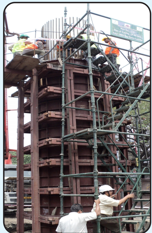
Construction of Metro Viaduct Pillar in Jokha - Mominpur Section of Kolkata Metro
