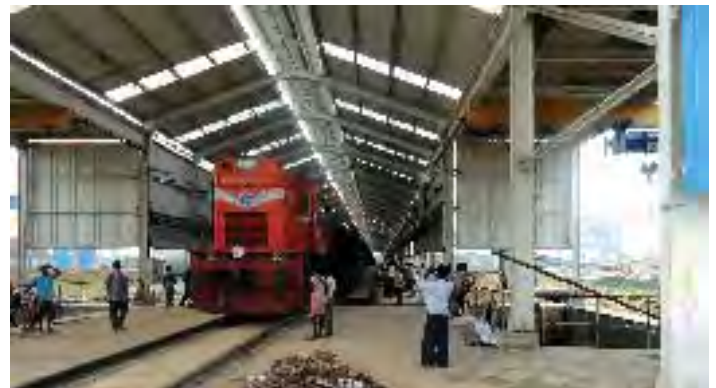
Commissioning of Track Hopper for unloading coal rakes at DSTPS Power House of DVC at Andal, West Bengal
