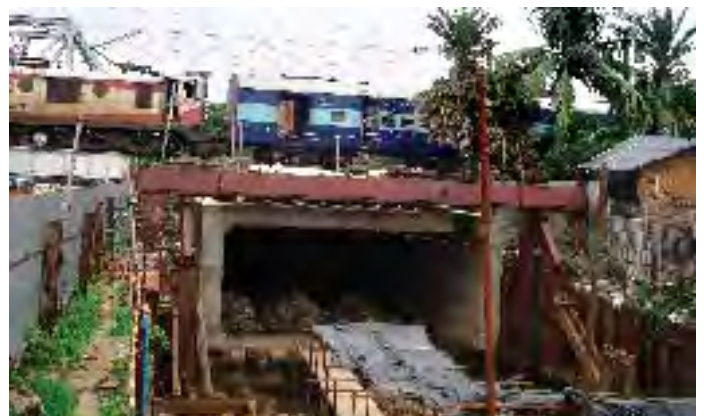
RCC Box Pushing work of KMDA at Patipukur below Quadruple suburban Railway track near Sealdah
