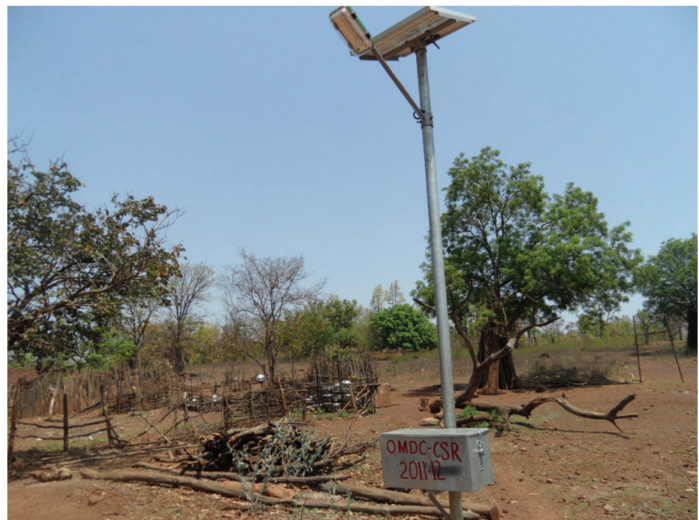
Street lights provided by OMDC under CSR Scheme.
