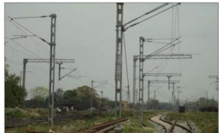
OHE, SAIL steel plant, Rourkela
