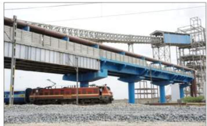
Bridge for Coal Conveyor and CW pipe line across Ennore Creek, Buckingham canal and Railway track for Vairur Thermal Power Project
