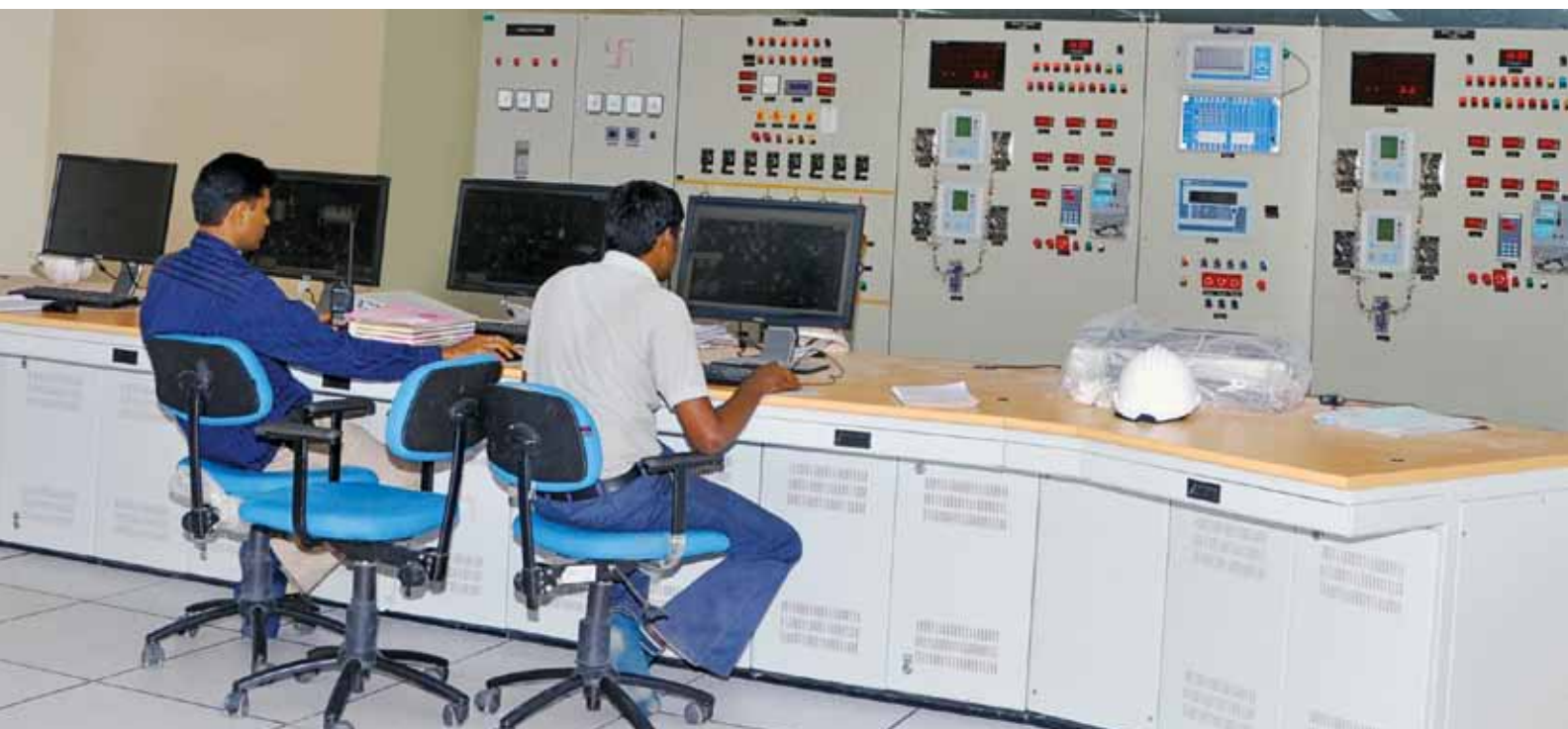
Cement Control Room, Ariyalur
