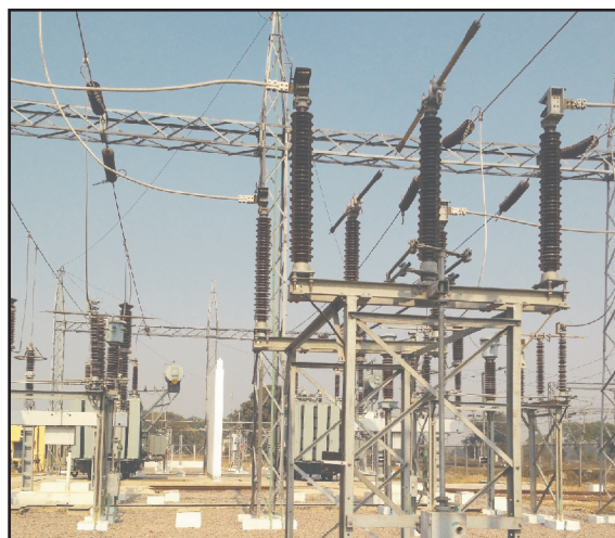
Sub-station in Lucknow-Mughalsarai Railway Electrification project
