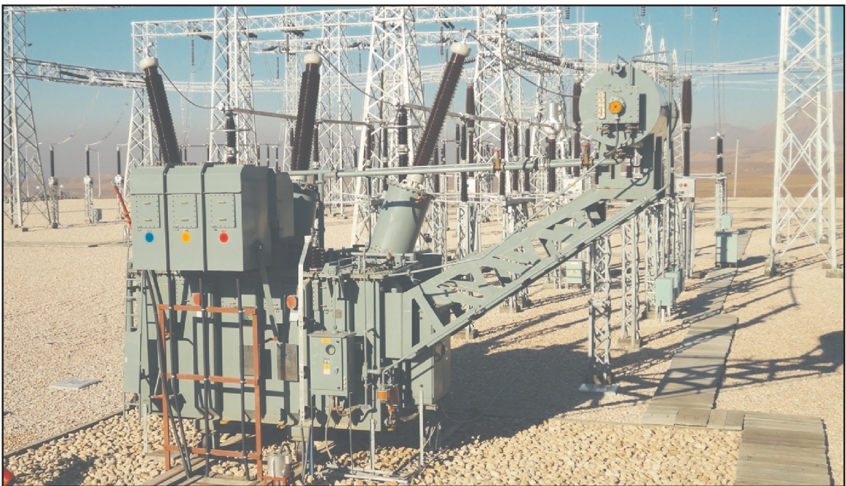
16MVA Power transformer at Aybak sub-station, Afghanistan
