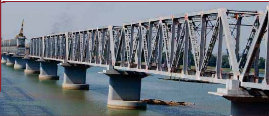
Launching of 92m Steel Girder over River Mahanadi Near Naraj in Rajatgarh Barang Doubling Project
