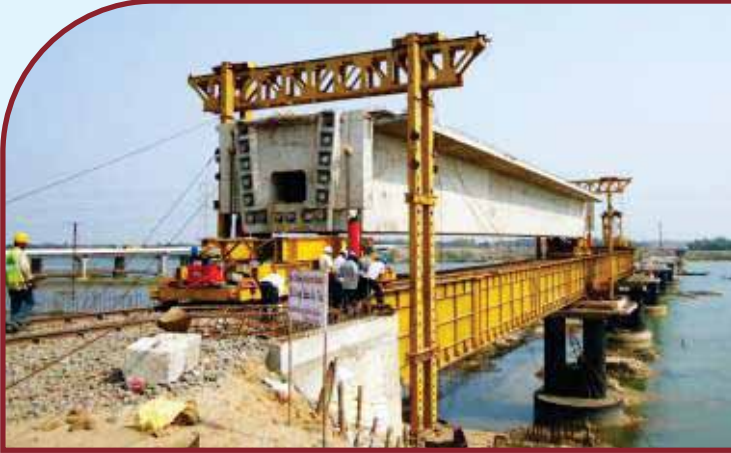
Launching of 600 Tonnes PSC Girder on Luna Bridge in Haridaspur Paradip Project
