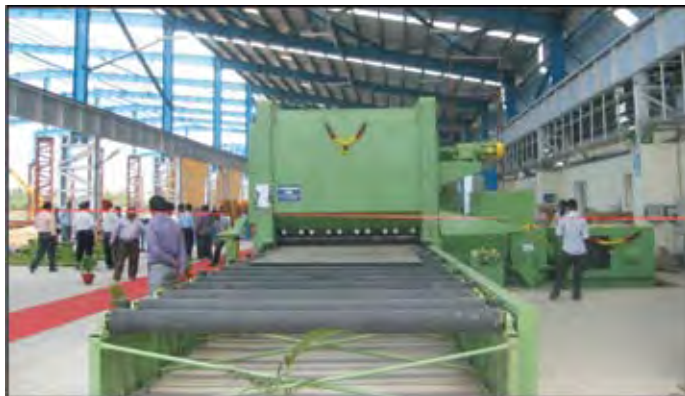
Turnkey work for FIAT Bogie Shop at ICF, Chennai: Installation of Plate Straightening machine
