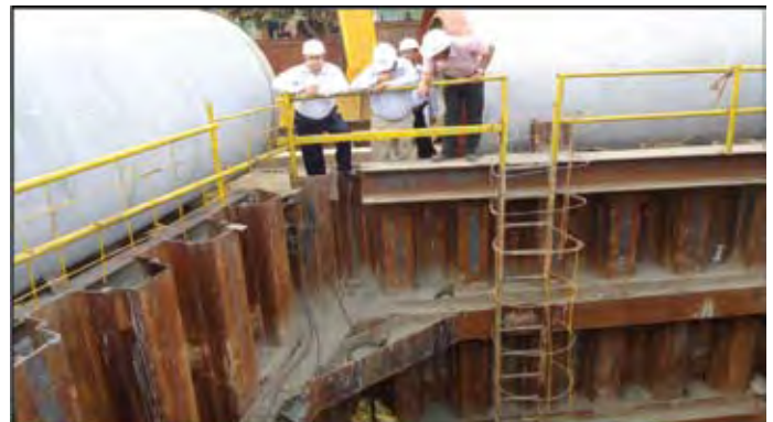
CMD Shri Rajeev Mehrotra and other officials inspecting the site of Tallah-Palta Dedicated Transmission Main, Kolkata
