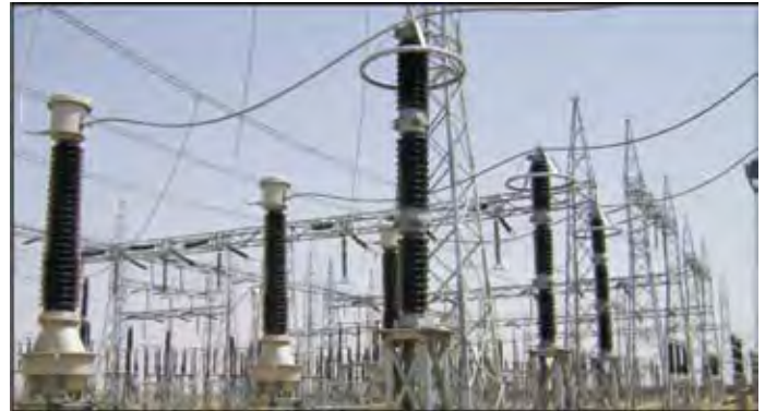
Sub-Station for Wind Energy
