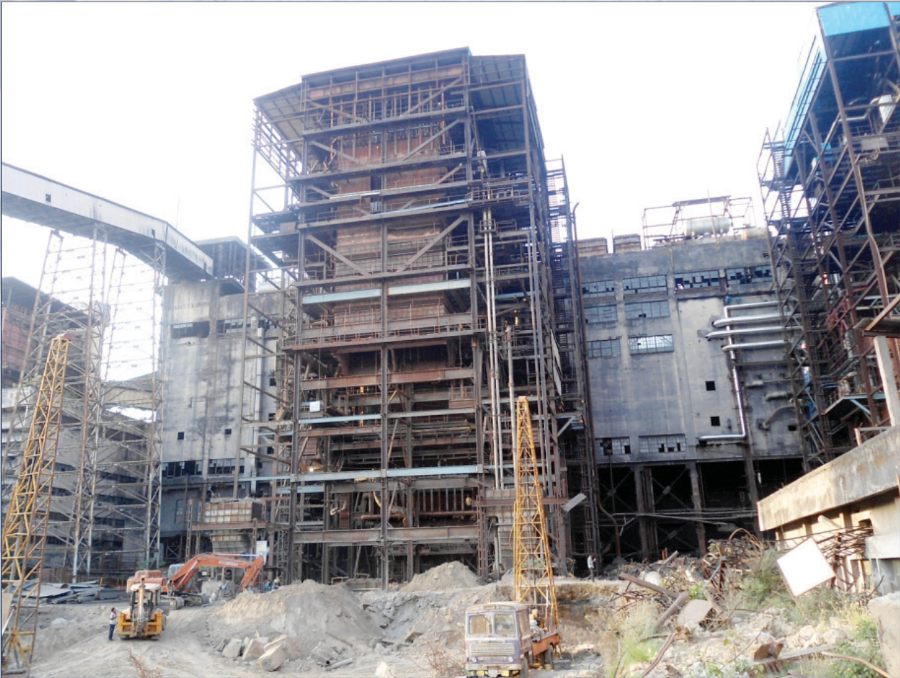
Baranu TPS Boiler V#6
