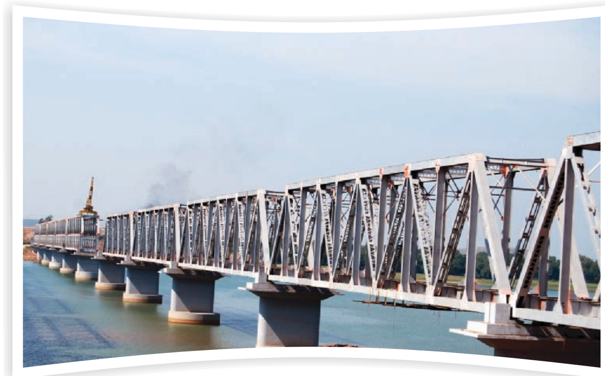
92 m steel through girder launching over river Mahanadi near Naraj in Rajatgarh-Barang doubling project.
