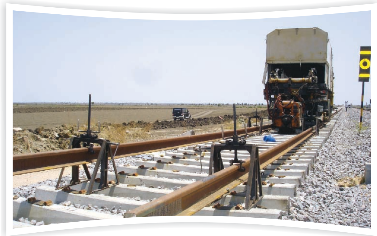
Ballast Spreading through Rail lorry in Section of Hospet - Tinaighat Doubling Project
