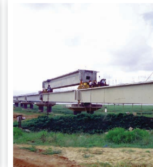
43.8 m PSC box girder weighing 650 tons launching over river Luna in Haridaspur - Paradeep NL project.
