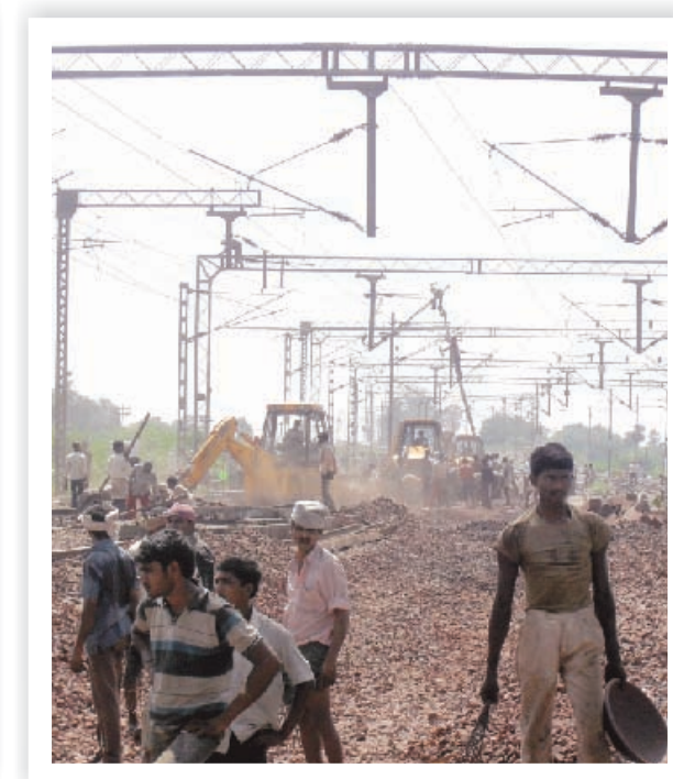
Non - Inter lock working in Gooty - Pullampet doubling Project
