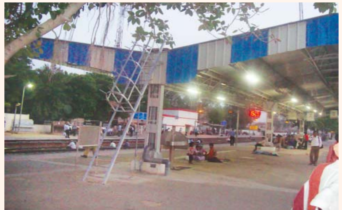
25kw Solar Power Plant on Platform shelter at Gurgaon Railway Station under CSR
