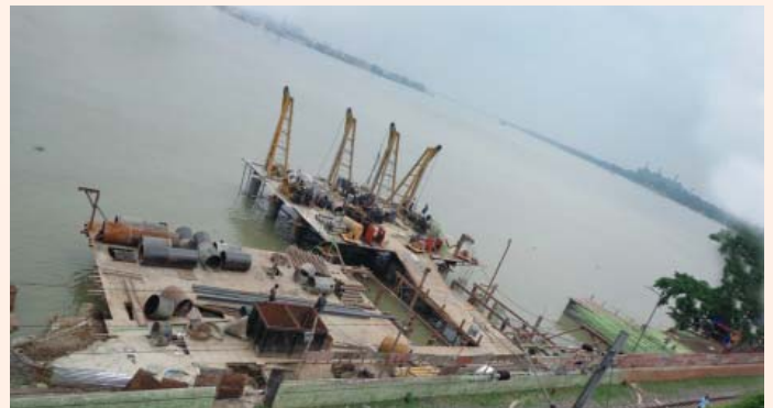
Intake Facility (Jetty) at Bagh Bazar, Maerghat Kolkata - KMC
