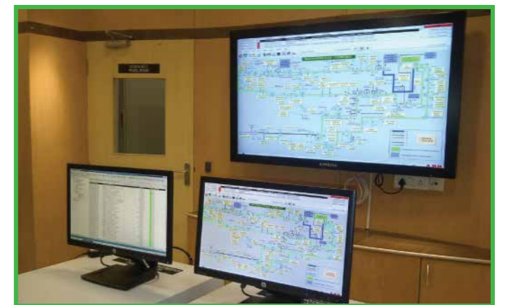
Effective monitoring - SCADA Control Room.
