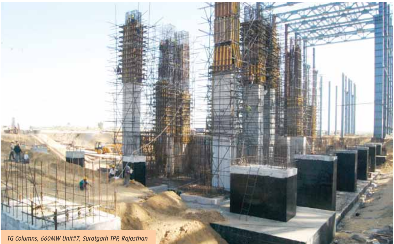
CW pump house Motor floor slab at 2 x 800MW, YTPS Project at Raichur
