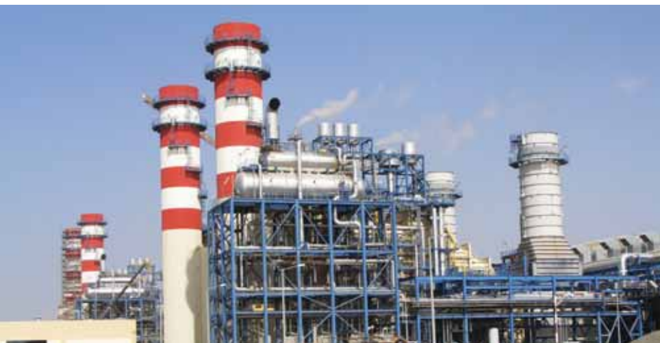
2 x 157MW Power Project, Libya
