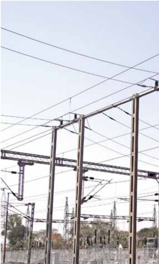
Railway Electrification PIU Bhopal
