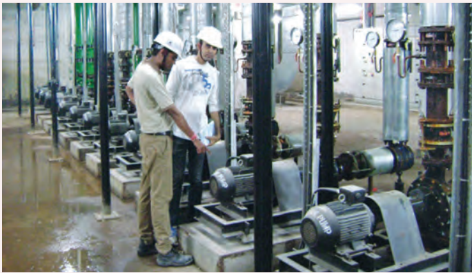
ILBS air cooled chiller plant
