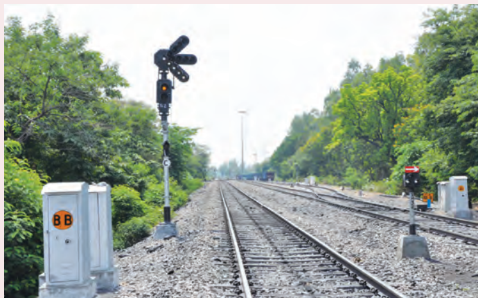
Route Relay Interlocking at NTPC, Vindhyachal (MGR)
