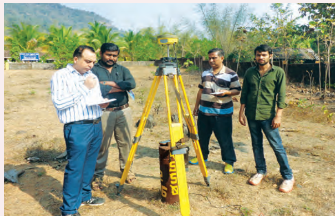
Fixing of ground control points with DGPS between Hubli and Madgaon for Southern Dedicated Freight Corridor
