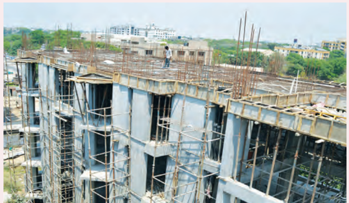
Construction of a Preventive Health Care and Skill Development Training and Research Institute for Santhigiri Ashram, New Delhi.
