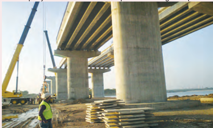
Work Zone Safety Audit by RITES Road and Bridge Safety Audit Team at the Mahi River Bridge on Ahmadabad to Godhara Section of NH-59
