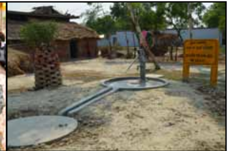
Hand pump along with Water Harvesting facility installed at Hariharpur, Korwa
