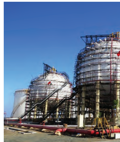
New LPG spheres at Pipavav commissioned in March 2016
