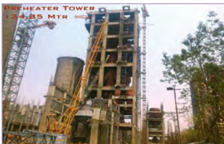
Preheater tower under mechanical erection at Manikgarh Cement Unit II, Gadchandur, Dist. Chandrapur, Maharashtra
