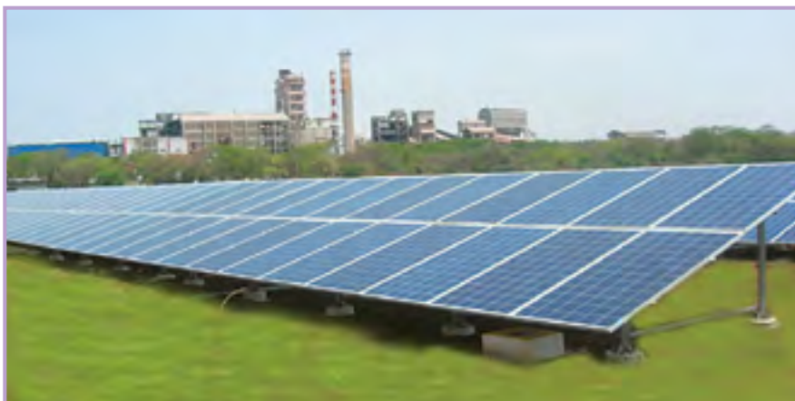
Solar photo voltaic power generation plant of 600 kw peak capacity at Century Cement, Baikunth, Dist. Raipur, Chhattisgarh
