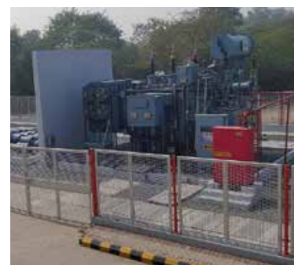
Commissioned 66/11 KV GIS Substation along with 2 x 31.5 MVA transformer at BRPL, Sangam Vihar
