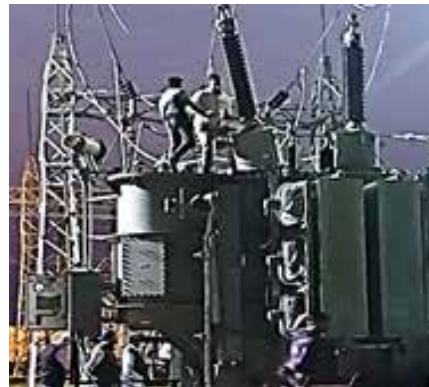
Commissioned 40 MVA, 132/33 KV Power Transformer supplied to PTCUL, Padartha
