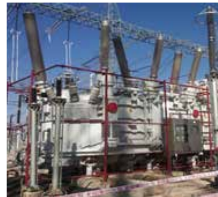
Commissioned 500 MVA 400 KV Auto Transformer at PGCIL Badla
