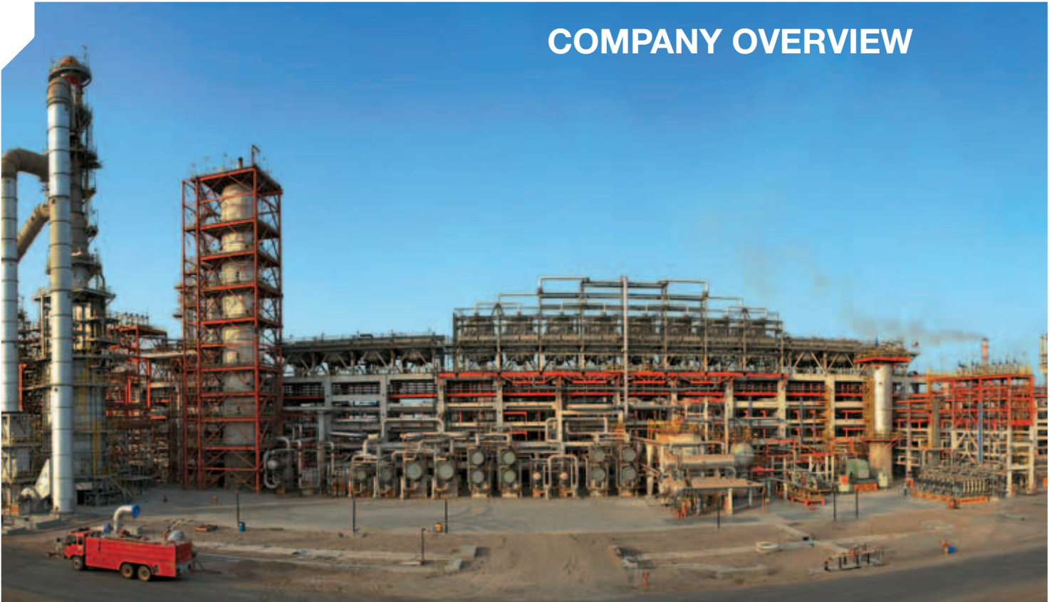
> DIESEL AND GASOIL HYDROTREATER UNITS AT VADINAR
