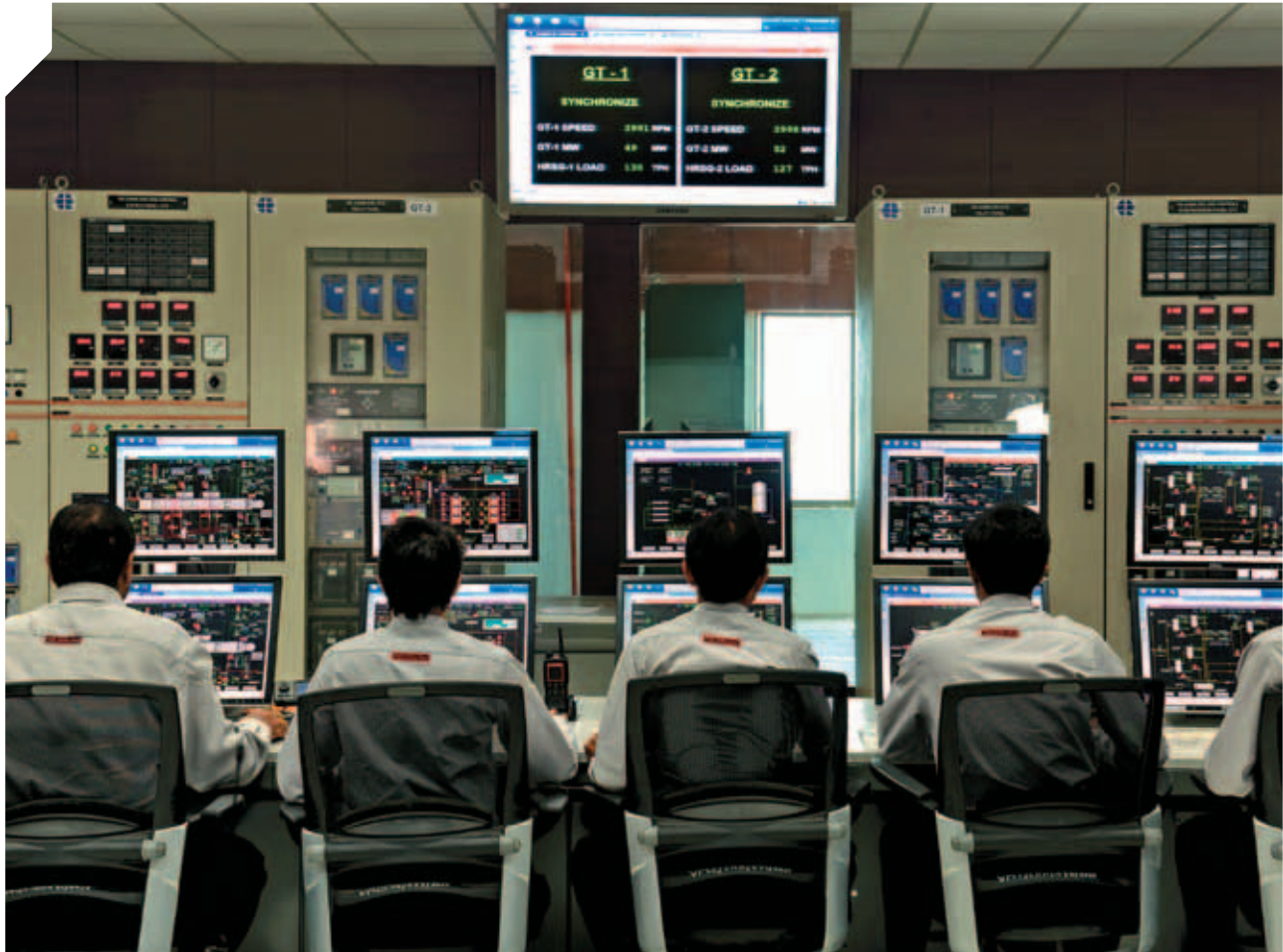
> CONTROL ROOM OF THE POWER PLANT AT VADINAR
