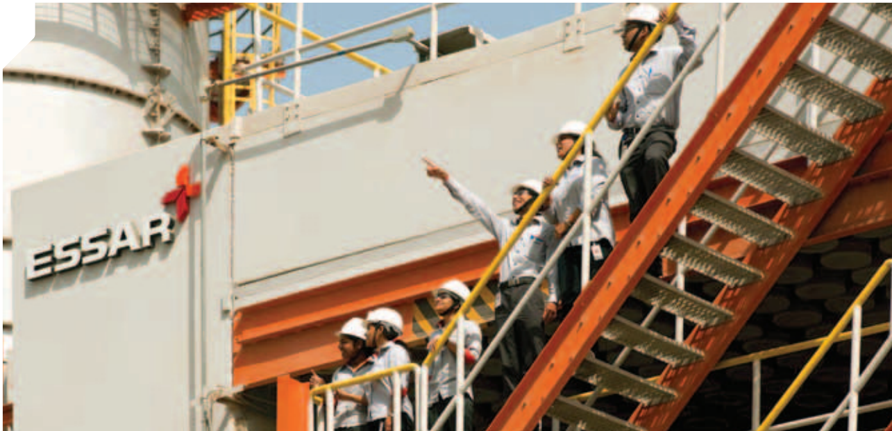
> UTILITIES AREA AT VADINAR
