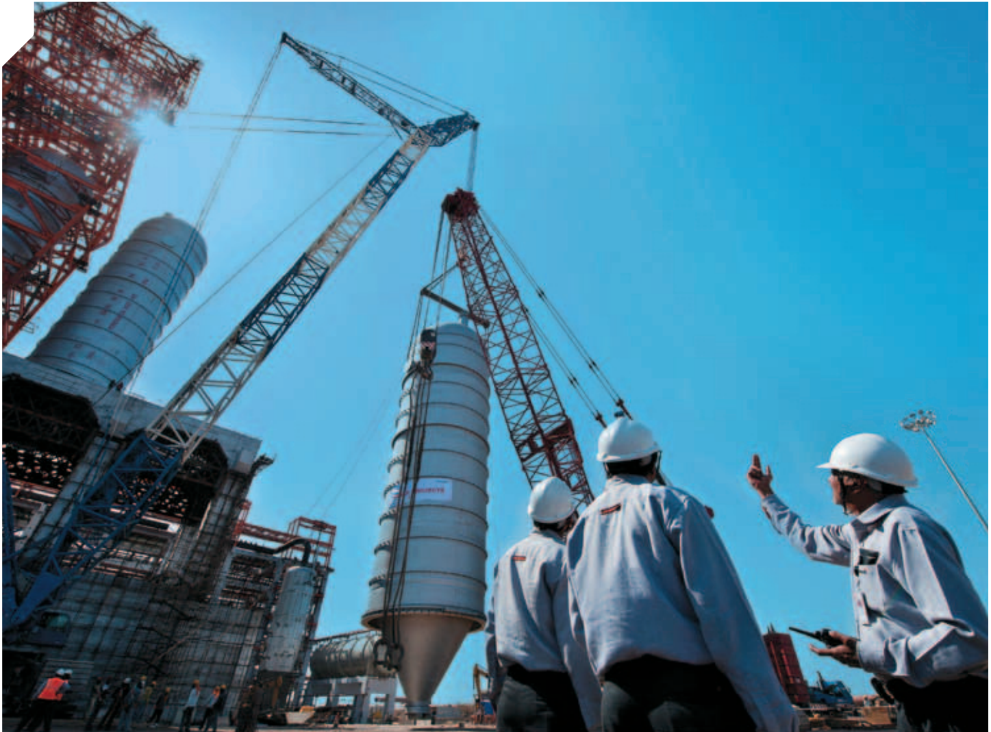
> DELAYED COKER UNIT AT VADINAR
