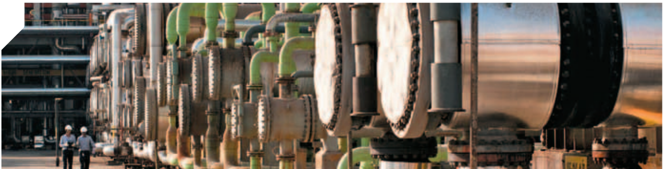
> A SECTION OF THE CDU AT VADINAR
