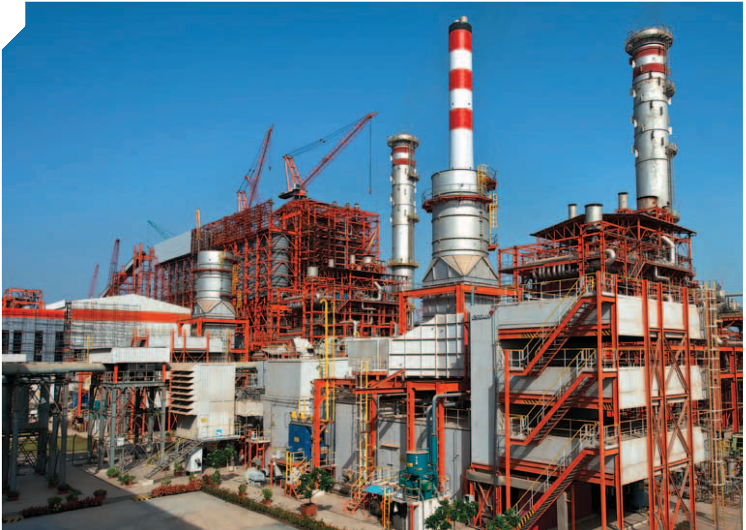
> POWER PLANT AND UTILITIES AT VADINAR
