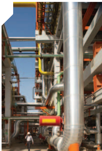
> A SECTION OF THE CDU AT VADINAR
