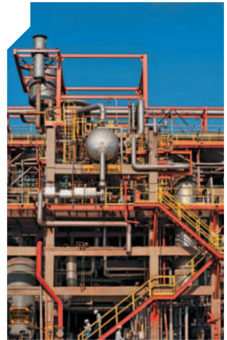
> A SECTION OF THE CDU AT VADINAR
