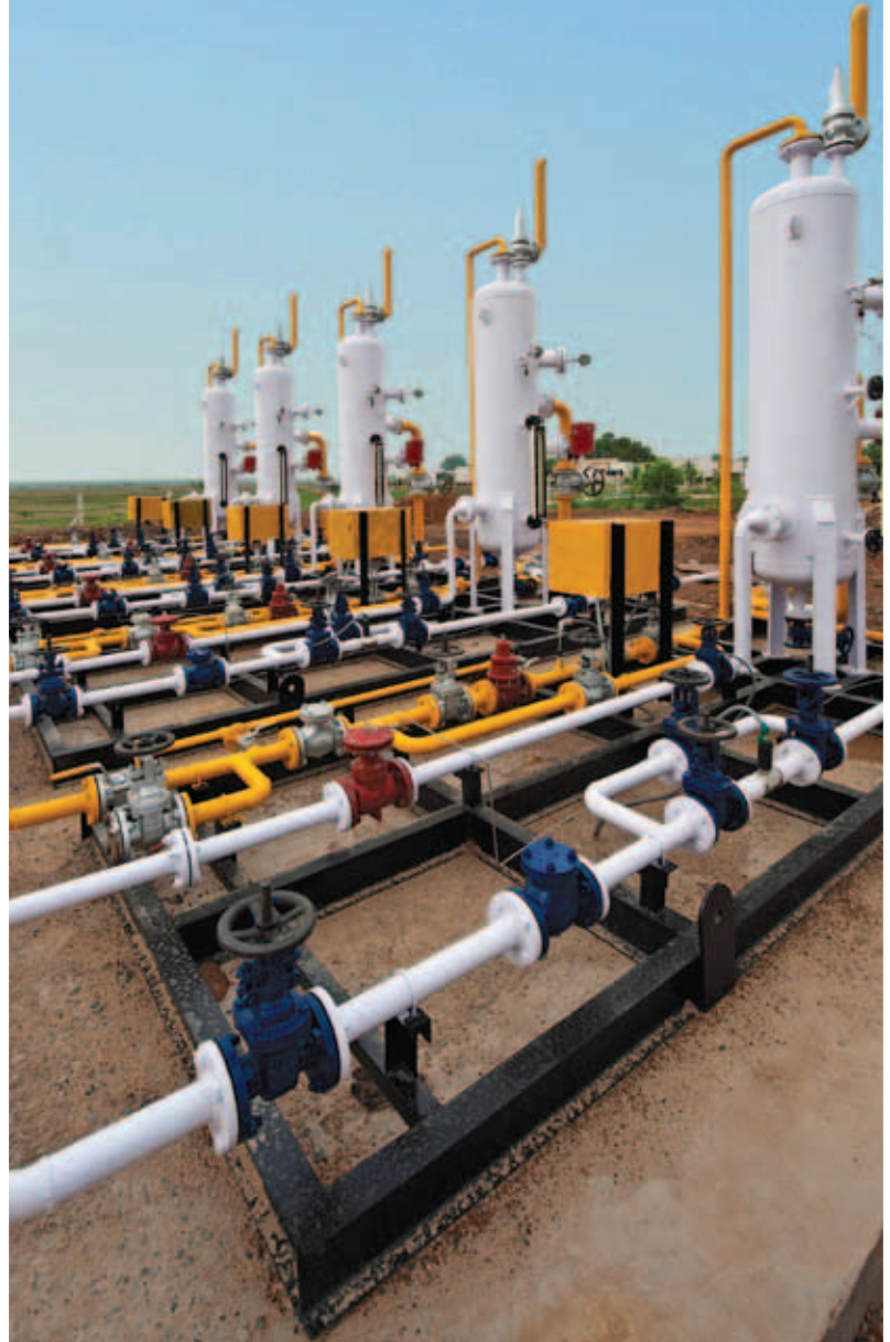
> SKID SEPARATOR AT RANIGANJ
