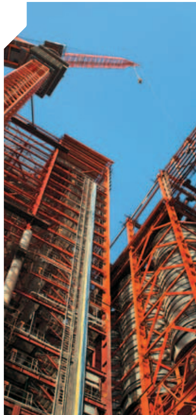
> DELAYED COKER UNIT AT VADINAR
