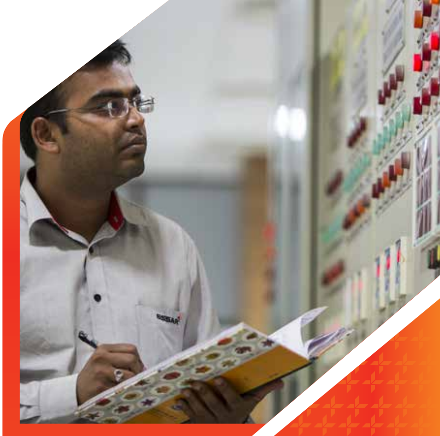
Coal-fired captive power plant Control Room at Vadinar
