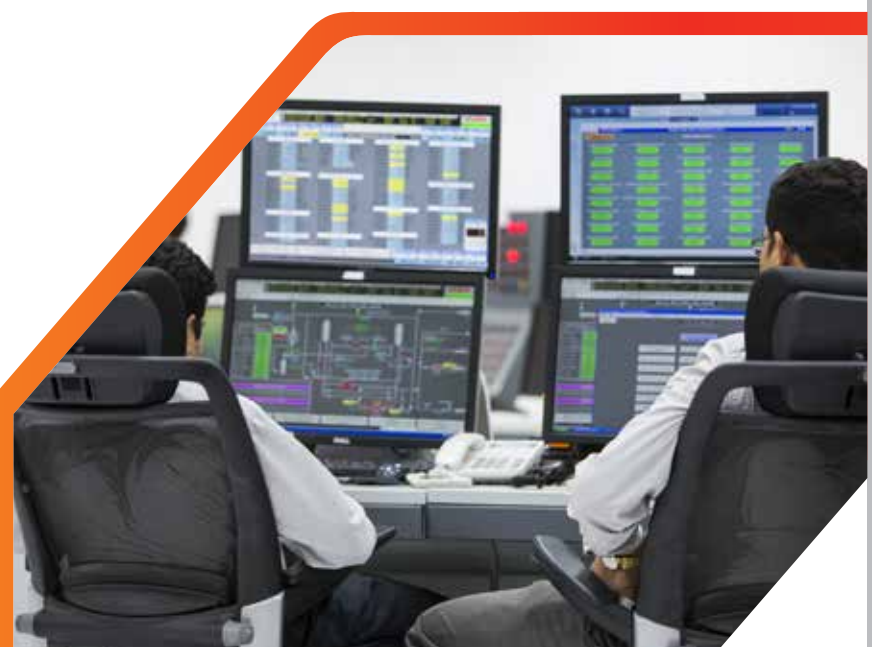
Central Control Room at Vadinar
