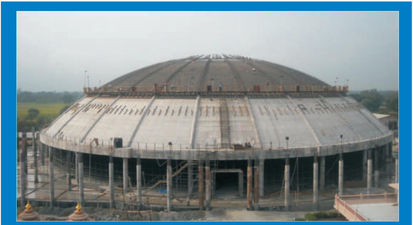
Design, Manufacture, Supervision for Erection of Scaffolding for Dome with Diameter of 82m & height of 32m at Pratapgarh, U.P.
