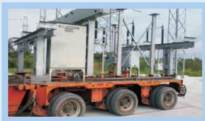
Supply of Mobile Sub Station- PHCN, Nigeria
