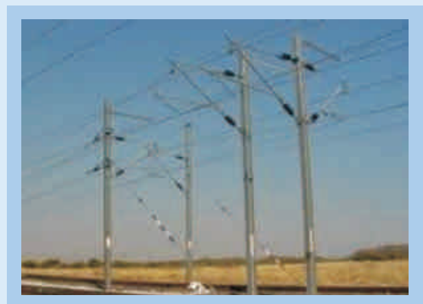
Over Head Electrification for Railways
