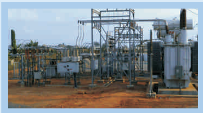
161/34.5 KV Mallam Sub Station-Ghana
