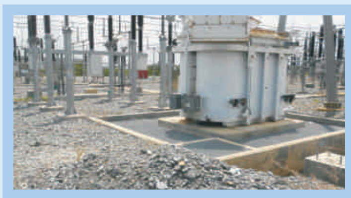
5MVA Power Transformer Installed at Kumasi Sub Station- Ghana
