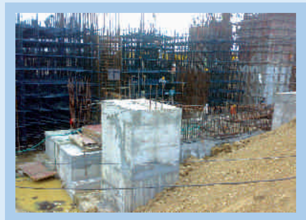
Koradi Power Plant, Nagpur
