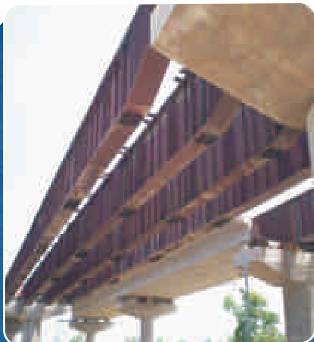
Complete fabrication and installation of 55m clear span Railway Over Bridge at Moradabad-Bareilly highway
