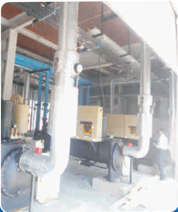
Commissioning of HVAC chiller plant of 600 ton at IIM-Noida
