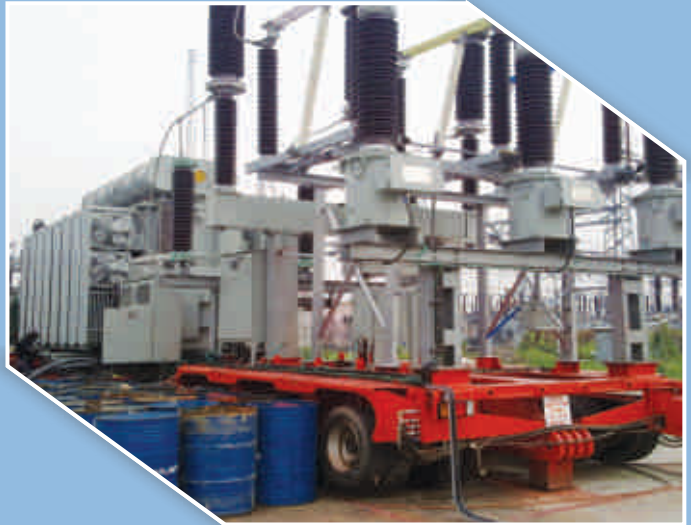
Mobile sub-station supplied to Power Holding Company of Nigeria
