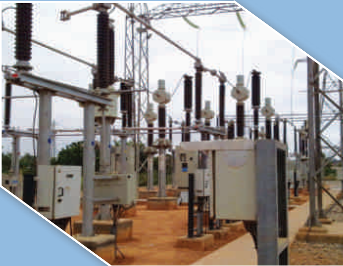
Mallam Sub-Station supplied to Gridco, Ghana
