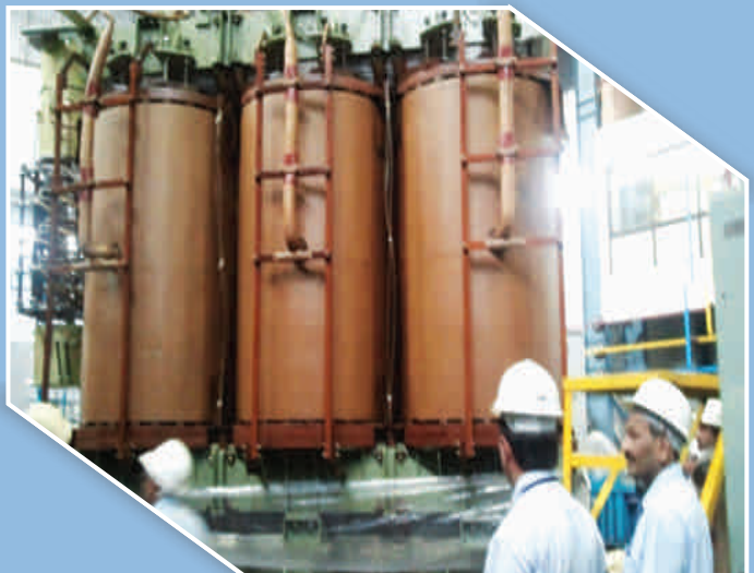
Power Transformers supplied to Volta River Authority, Ghana
