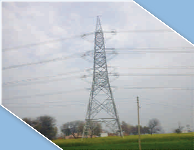
EHV (Extra High Voltage) Transmission Lines
