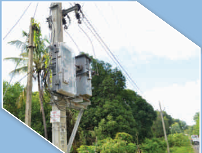
HVDS (High Voltage Distribution System) Projects
