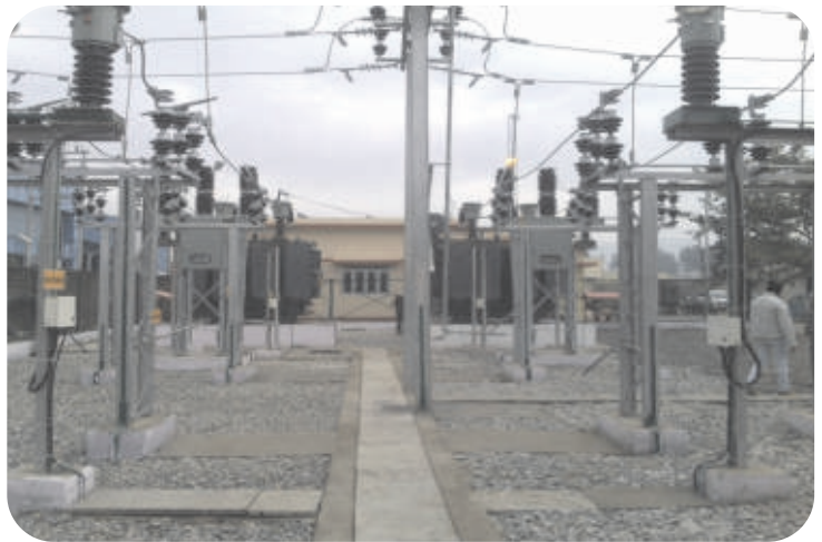
33/11kV Selaqui Substation
