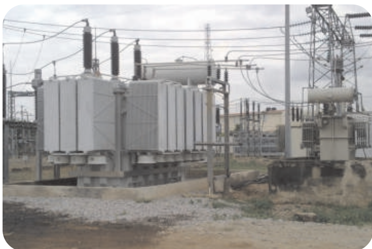
Ayede 330/132/33kV sub-station
