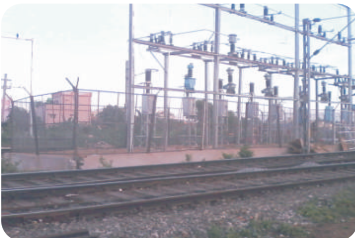
Overhead Electrification for Railways
