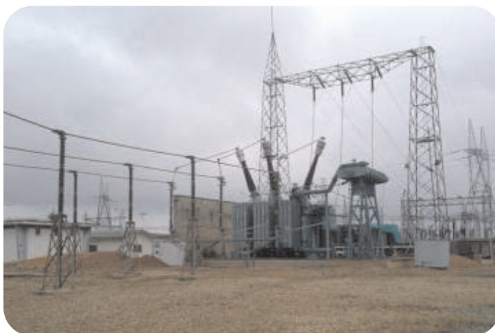
330/132/33kV transmission sub-station, Power Holding Company of Nigeria
