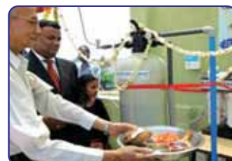
Drinking water purification plant installed at SOCARE, being put into operation by Mr. D. G. Rao, Chairman, and Mr. Dinesh Sadasivan, ED & CEO, of Ion Exchange Services.
