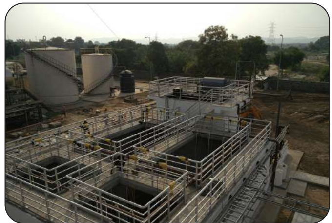
Complete ZLD System for a leading Brewery
