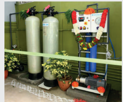
Demo plant for vocational training, Shishu Mandir, Karnataka
