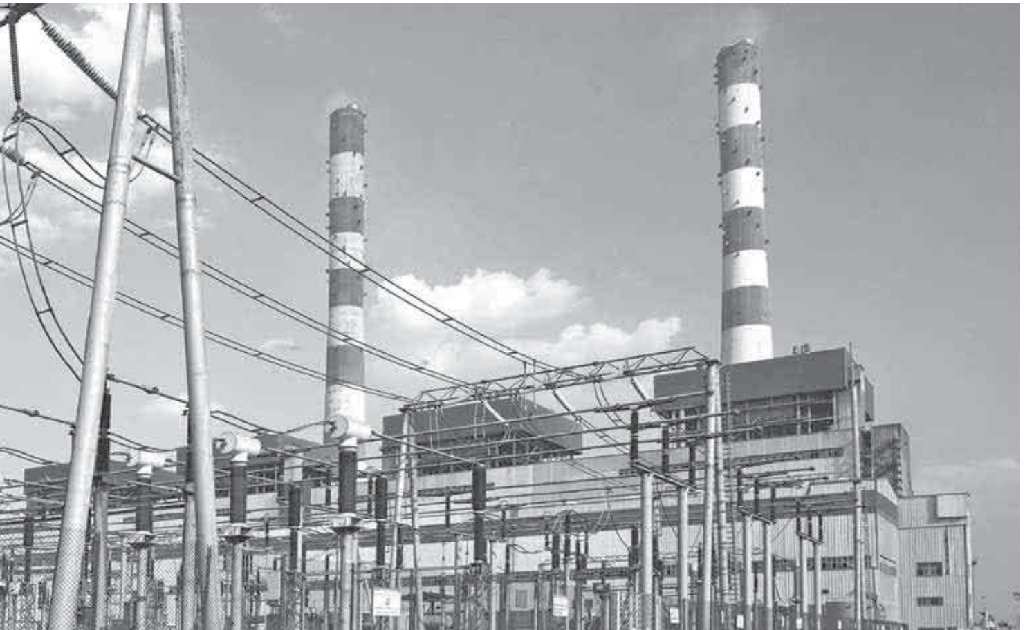
BALCO power plant
