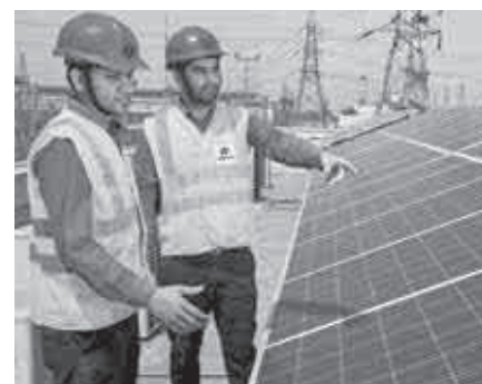
Solar panel installed in comprehensive building, BALCO
