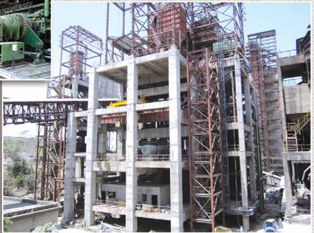
The Roller Press Building at Durgapur Cement Works, Durgapur, West Bengal; (inset) the newly commissioned Roller Press
