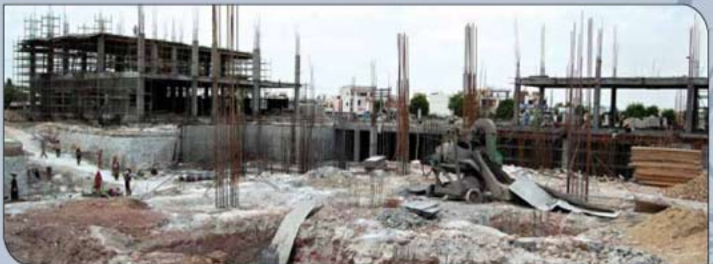
A view of the M P Birla Hospital & Research Centre, under construction at Chittorgarh, Rajasthan
