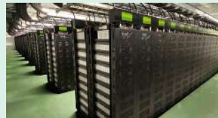
ENERGY STORAGE/ LITHIUM-ION BATTERIES
