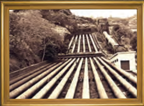
Pipelines to carry water to Power House
