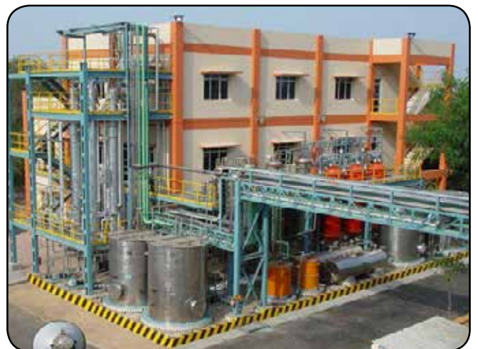
A section of the Fine Chemicals Plant
