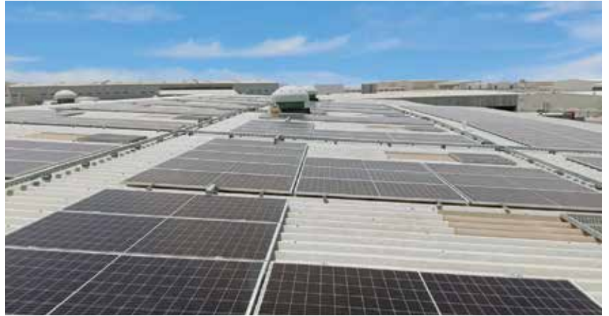
||||||| Voltas commissions first solar project in Dubai For SirajPower
