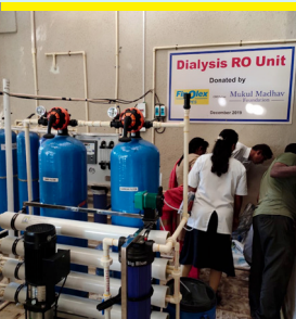
RO Unit at Civil Hospital Ratnagiri, Maharashtra
