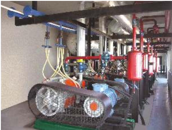
◀ Battery of KC KCX series compressors at EOU unit for food processing and preservation
