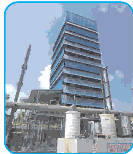
Phenol Recovery Plant
