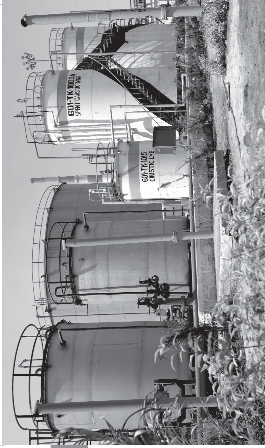
Chemical Handling System-HPCL
