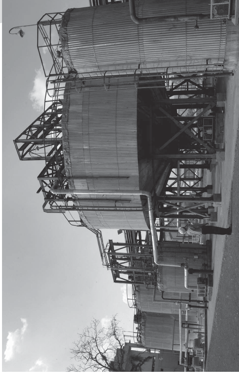
Causticisation Plant, Vedanta, Lanjigarh
