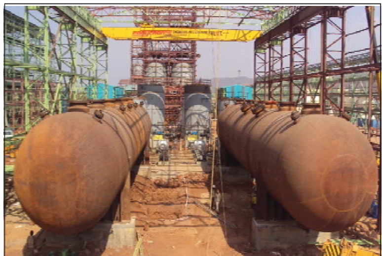
INCONEL CLADDED AUTOCLAVE - UCIL - Kadappa Site
