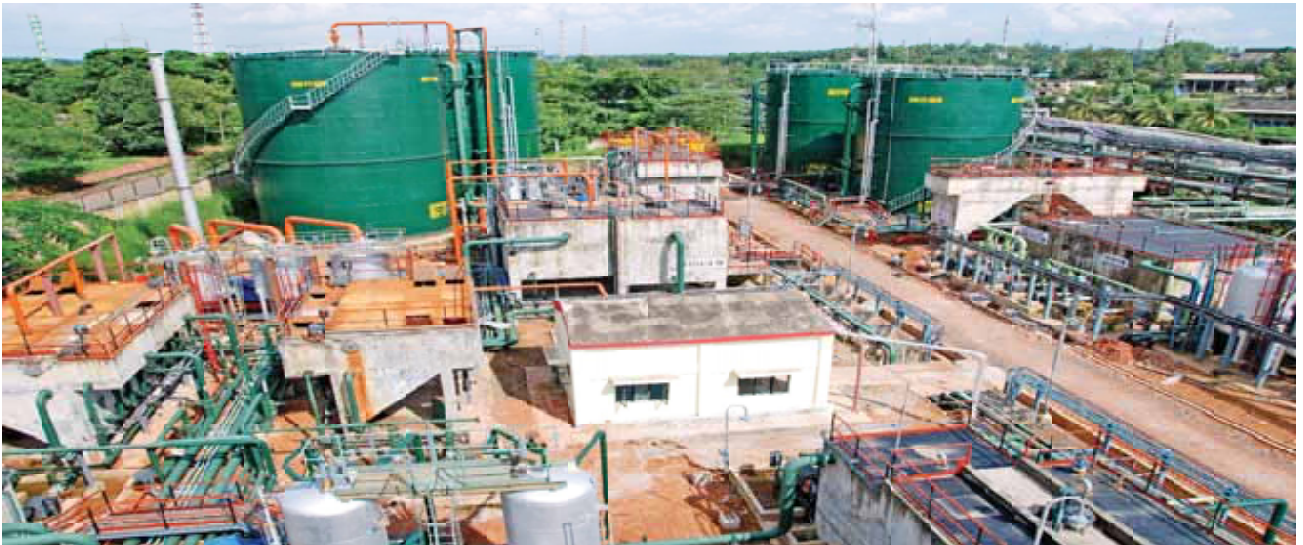
BPCL - KOCHI - Effluent Treatment Plant
