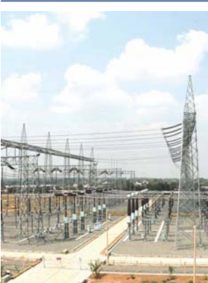
Solutions ranging from 66 kV to 1200 kV for both AC and DC network
